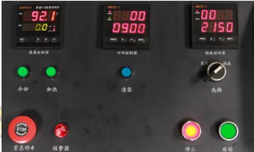
Fig.3 Electric cabinet and control panel
